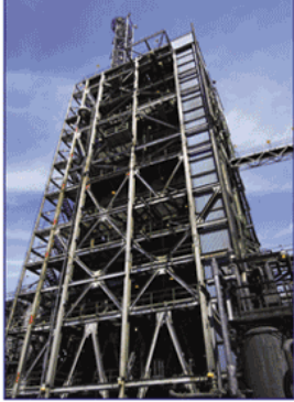
Nitrogen fertilizer gasifier in Coffeyville
